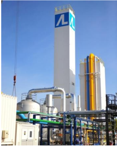
Air separation unit
